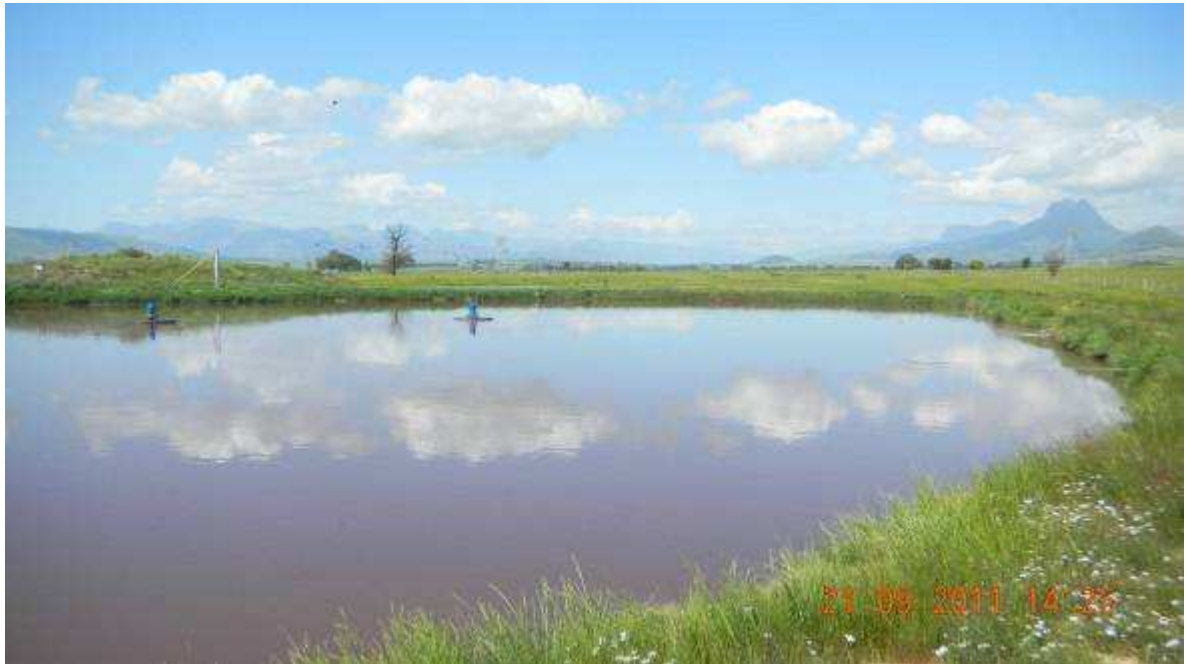
Figure 6: The existing treatment dam at Zandam with floating aerators.
