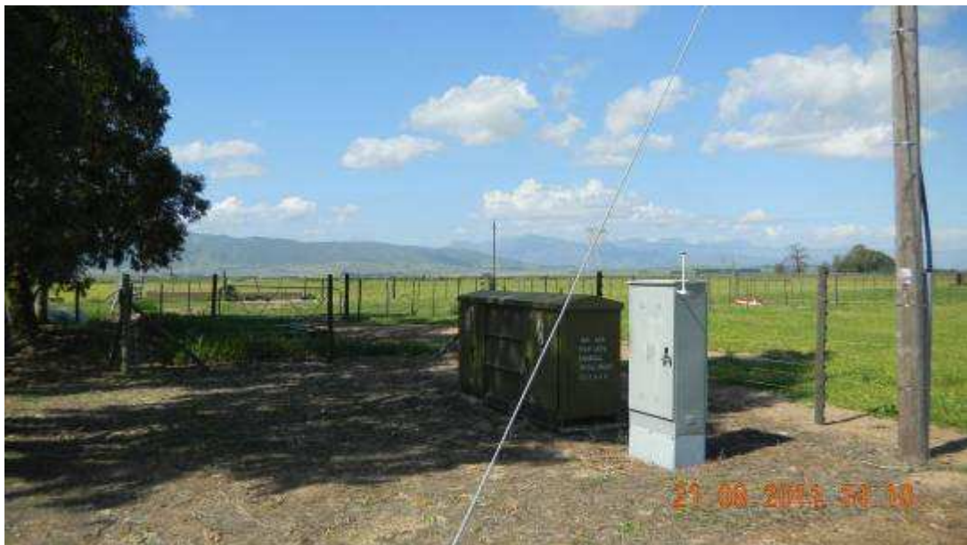
Figure 11: Electrical substation next to Digester site where connection to electrical grid will be done
