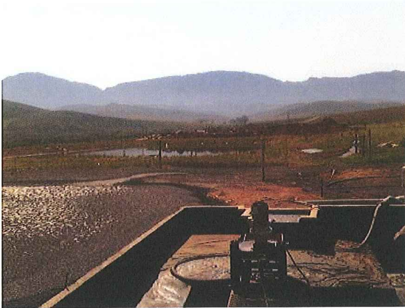
Figure 5: The existing treatment plant showing separator in foreground anaerobic pond on left and aerobic dam in background.
