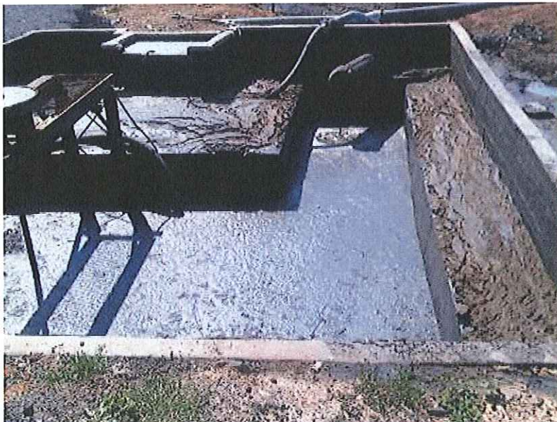
Figure 6: The existing separator.
